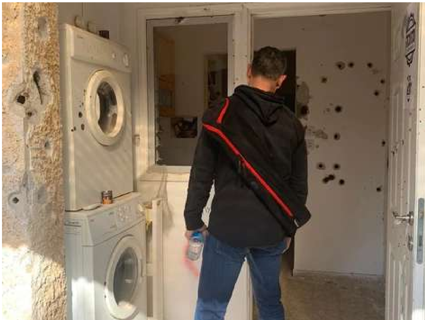
A visitor inspecting damage to house in Sha'ar HaNagev, Jan. 22, 2024. PHOTO BY ROB ROBERTS /National Post
