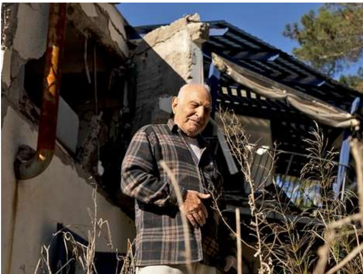
Kibbutz member Eli Mualem inspects a house that was hit by a direct missile during the war, as he returns to the kibbutz near the Lebanese border in Manara, Israel. PHOTO BY AMIR LEVY/GETTY IMAGES
